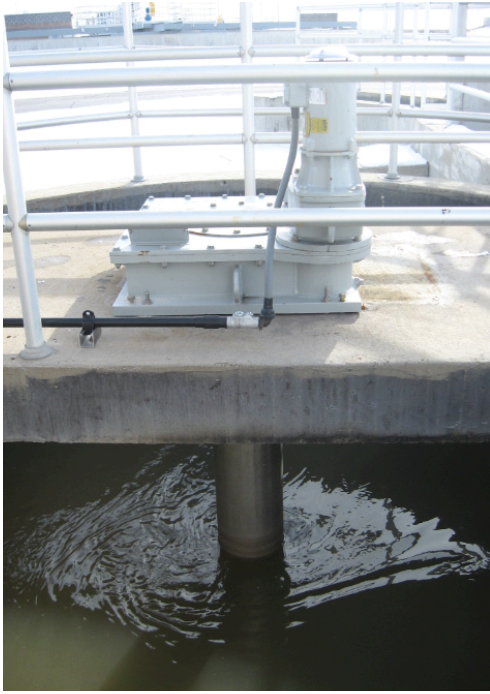
HDE provided a customized grit solution to fit an existing concrete chamber. (IMG_0043.JPG)
